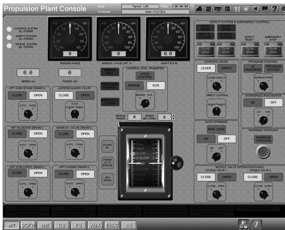
Fig. 1. Main turbine remote control panel
